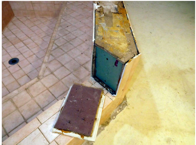
Plywood and drywall, really shoddy construction for such a wet area.
