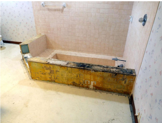
This part of the wall had the worst mold.
