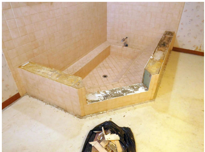
The entry section is all shorn of tile.
