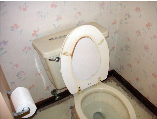
The 28 years with no maintenance showed in the toilet seat condition.
