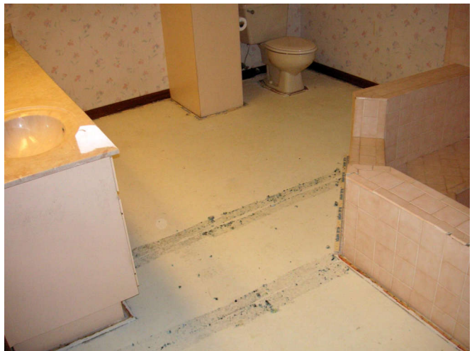
The bath area carpet nail strips are next. The glue lines get cleaned with acetone.
