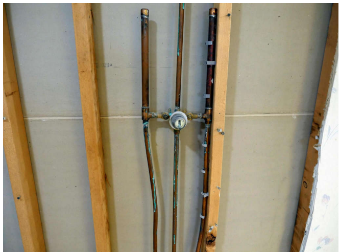
Unbelievably bad construction.
