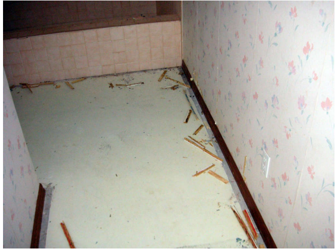
Here is the entry hallway with the carpet nail strips pulled up.
