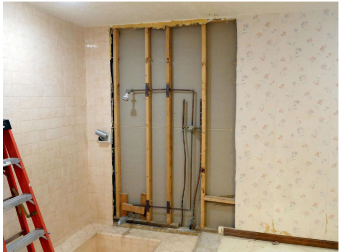
The water outlets are as bad as the valve.
