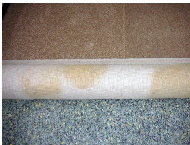
The dog pee stains were everywhere. The blue is the carpet underlayment mat.
