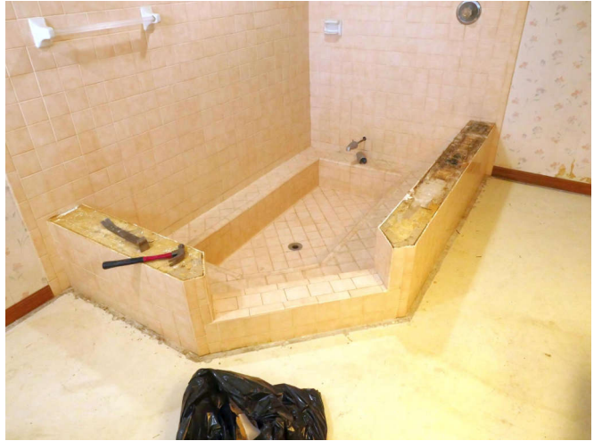
The tile was loose where the black mold is. I "encouraged" the rest to pop off, it didn't take much effort, a few tiles a day.
