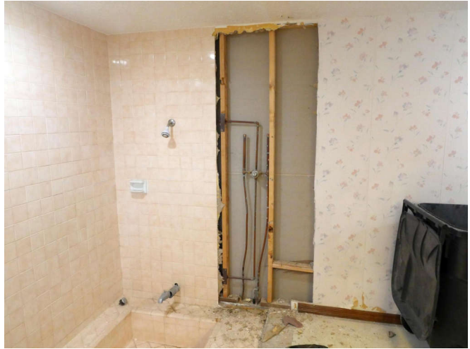
The shower valve is cobbled in a very sketchy method. Don't do this people.
