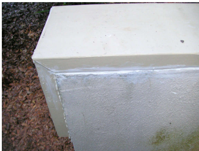
The residue from the old tube was just enough to seal the back side of the wall.
