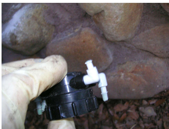
The little threaded part broke off in the tube. I call this collateral damage, friendly fire.
