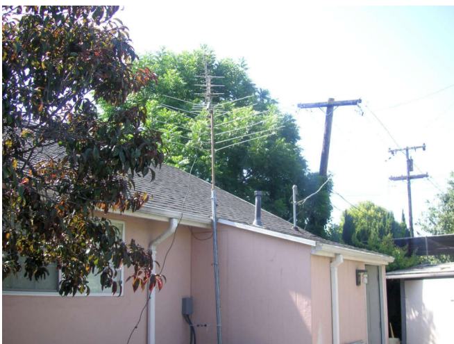
I gave the antenna mast & rotor to buddy Dave Mathis, and used a conduit in the meantime.
