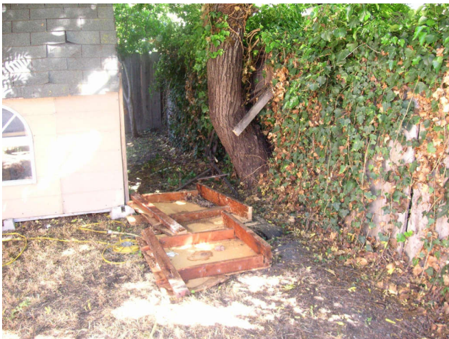
All that was left was to pry and unscrew the lumber from the shed.
