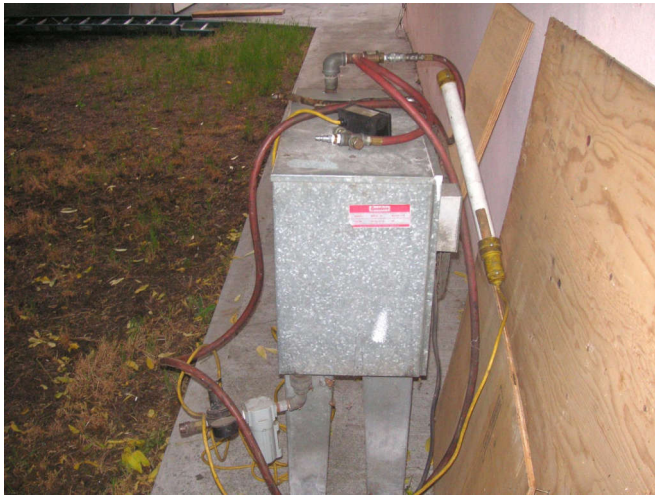
This is an air-to-air cooler for compressed air. It dries out the air for the bead blaster or painting.
