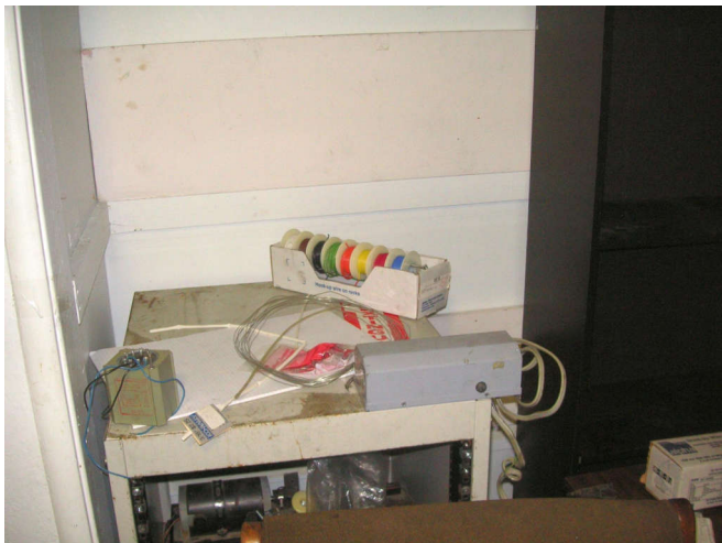
The hook-up wire made the move, as did the rack and the transformers.
