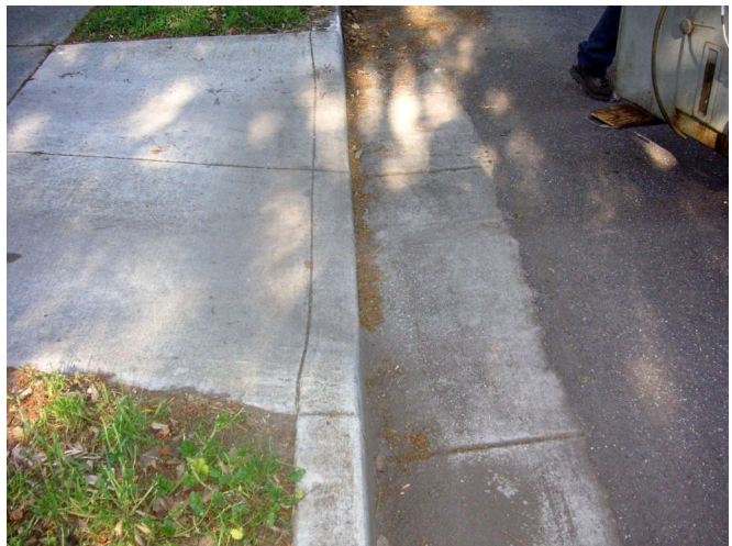
No cracks or damage on the curb cut, and the lather barely wiggled as they got it out.
