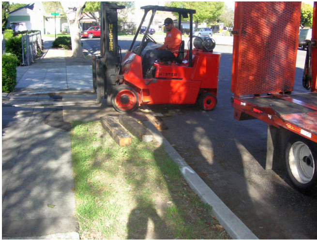
Rather than use my neighbors curve-cut like the guys that brought the mill, these guys used cribbing to jump the curb and a steel plate.
