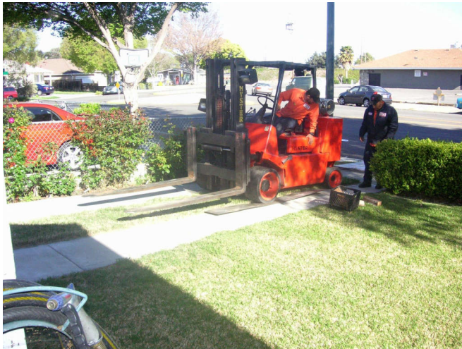
The concrete strips were almost too wide apart.
