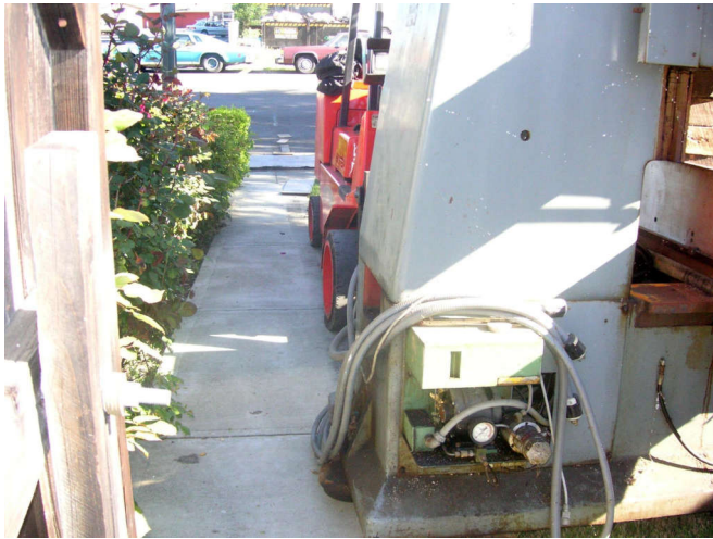
The tires have a little more concrete under them on this side of the machine. They have to get it past a gate you see in the foreground.
