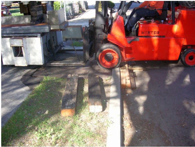
You can see how far out on the forks the machine is. Here is a movie clearing the curb..
