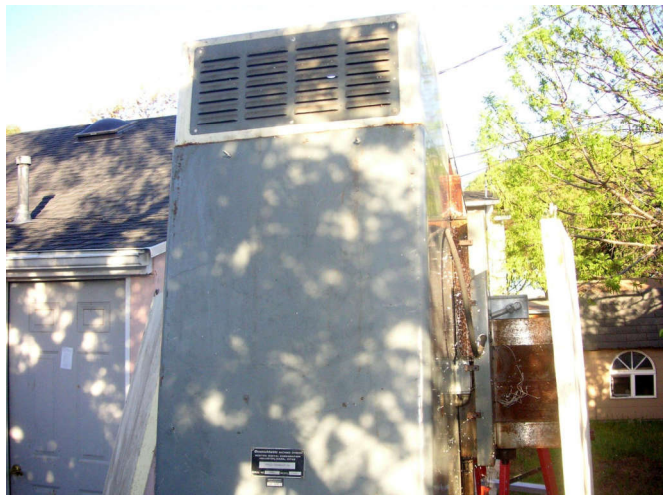
That top cover was so heavy, it was hard to lift. I guess they have gantry cranes at the factory.
