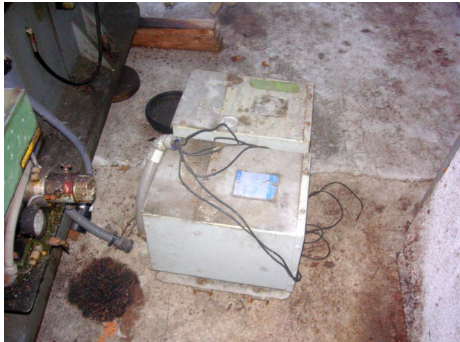
The machine came with this 208-to-240 Volt transformer. It was necessary to run the spindle motor inverters at 240 volts.
