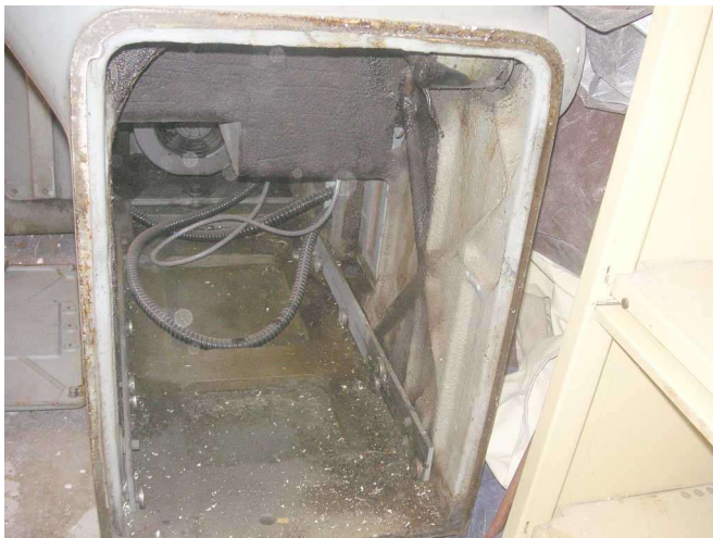
This is the area where the vacuum tube dc motor controller went. The ac inverter was mounted on the back, to keep cool.
