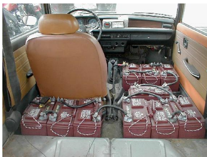
12V batteries with passenger seat removed.
